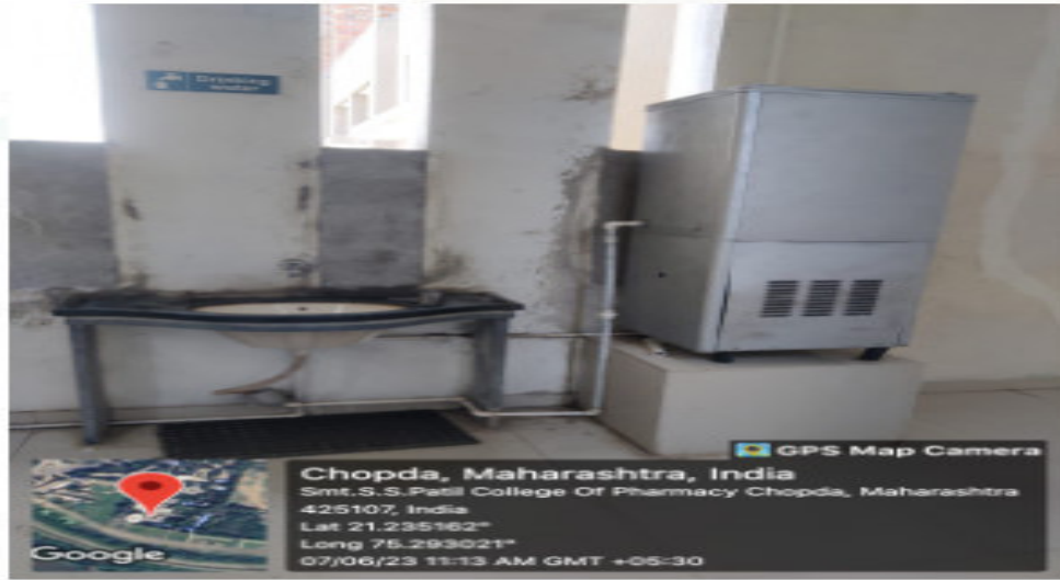
Drinking water Plant
