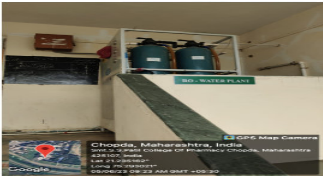
Water purification plant
